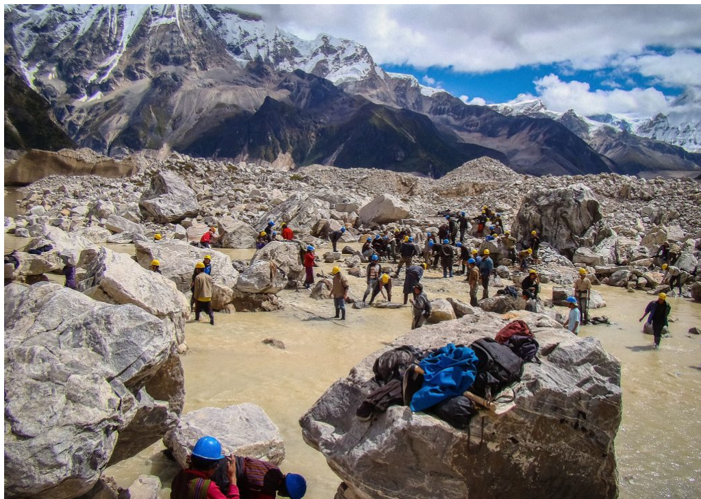
Figure 9. Lake lowering works at the dangerous Thorthormi lake were conducted by the Bhutanese government between 2008 - 2012 (Source: WWF)
